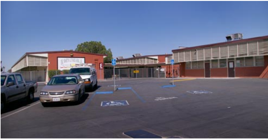
Site: chain link gates, directional signs, re-strip portion of parking stalls, accessible entrance/exit signs, wheel stops, accessible parking concrete, ramps in the path of travel, ADA signage
