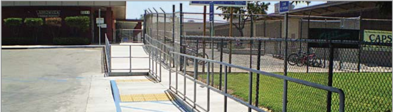
Arrowview Middle School Modernization ADA accessible walkways includes new concrete ramps and visual & tactile upgrades.
