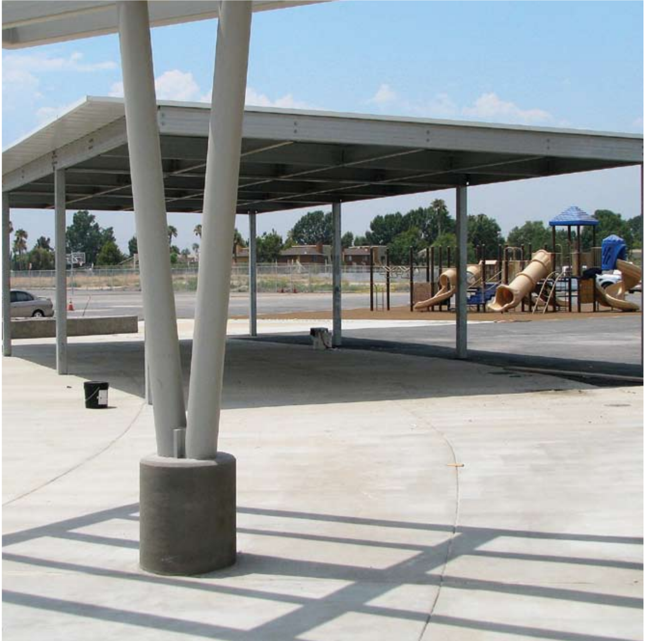
Wong Elementary School New Campus Lunch and shade shelter complete; play equipment installed.
